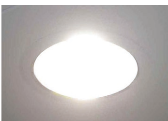
Original recessed lighting
